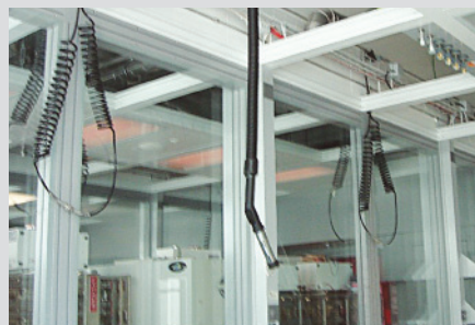
PHOTO OF ACTUAL RECOIL HOSE AND MANIFOLD MOUNTED TO WALL.
