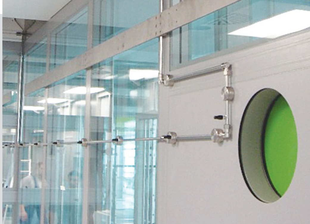
THE END OF THE INSTALLATION PROCESS WITH DRINKING VALVES CAPPED AND READY TO BE USED.
